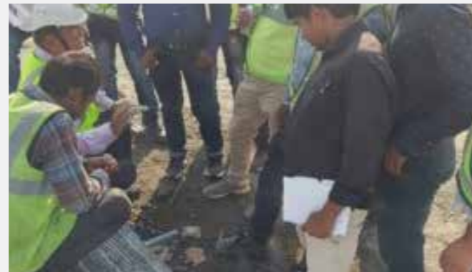
Rigid Pavement Construction Techniques Programme held at Mumbai Nagpur Expressway Project on Feb 14 th - 15 th , 2020
