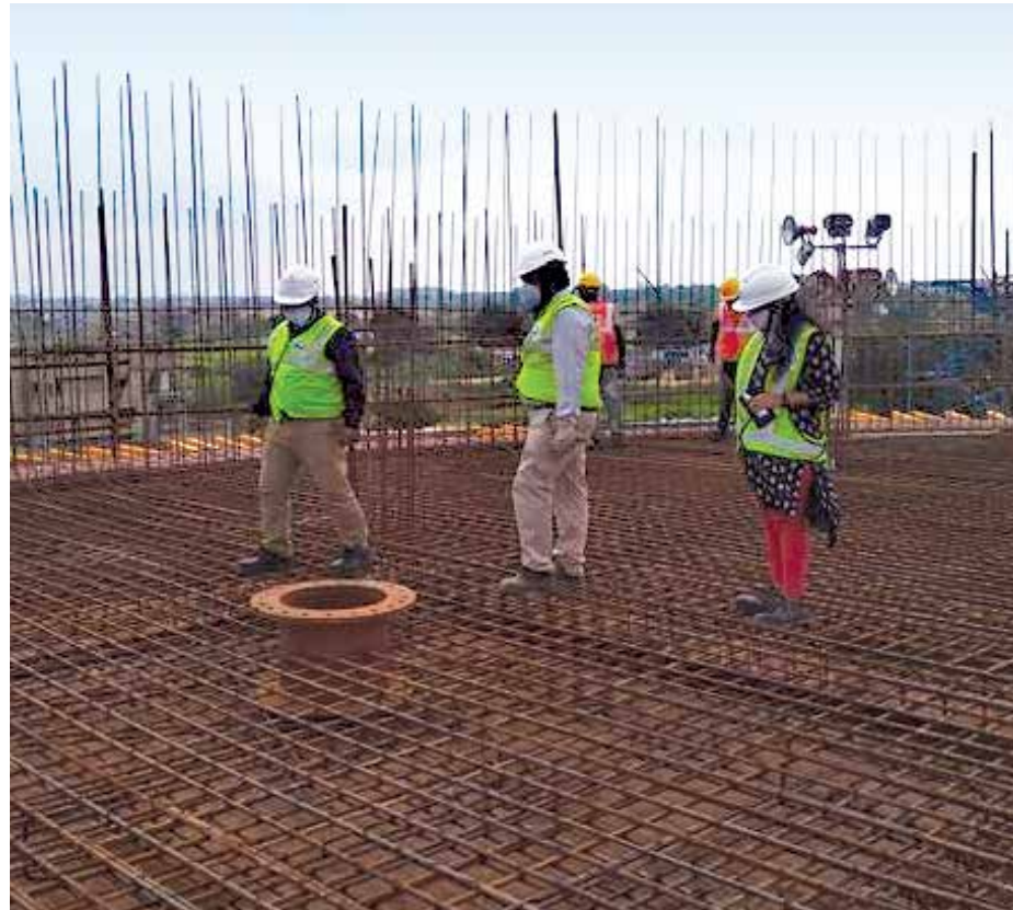
2.45 ML capacity Elevated Service Reservoir under construction at Ranchi WSS Phase-1 Project
