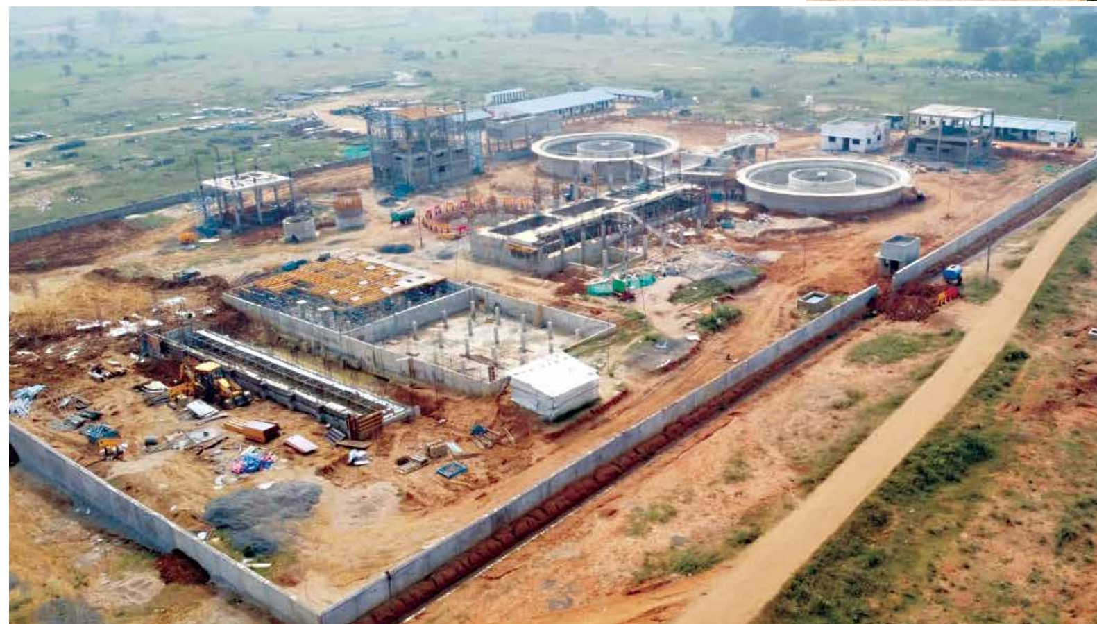
Overview of the 20.12 MLD Water Treatment plant under construction at RWS Boudh WSS Project
