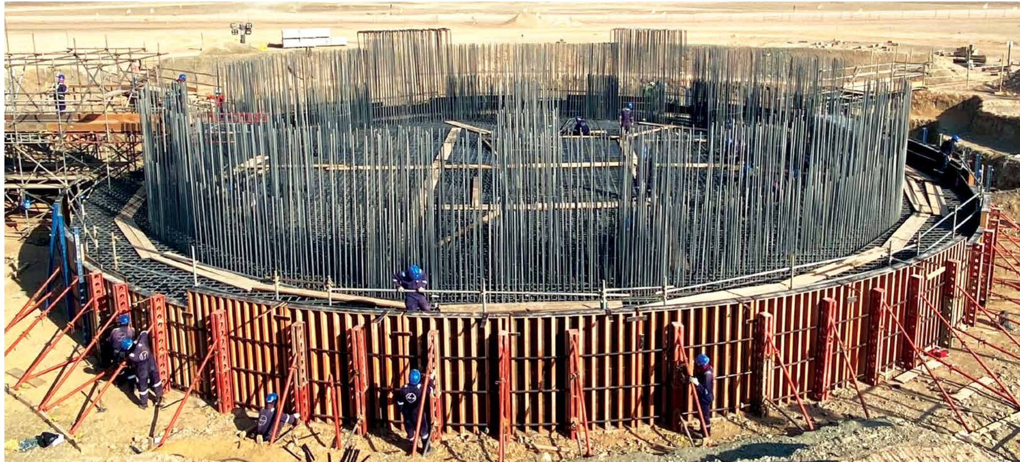
Crushed ore silo at MMGP
