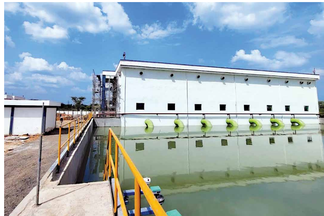
A fully operational pumping station at Bhalak
