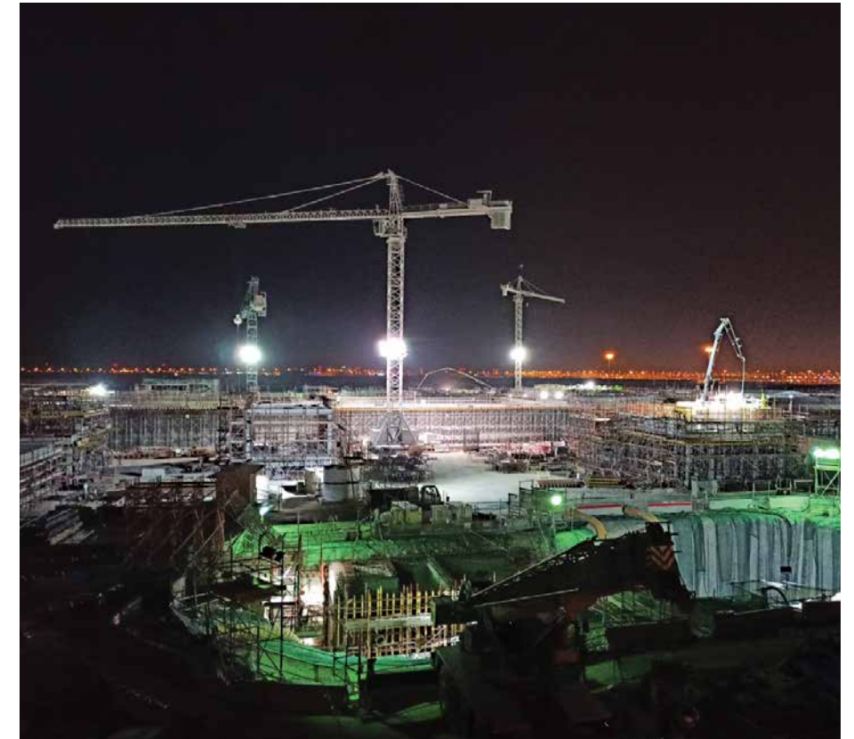
Night operations at the Industrial Area Sewage Treatment Works, Phase 3A Project
