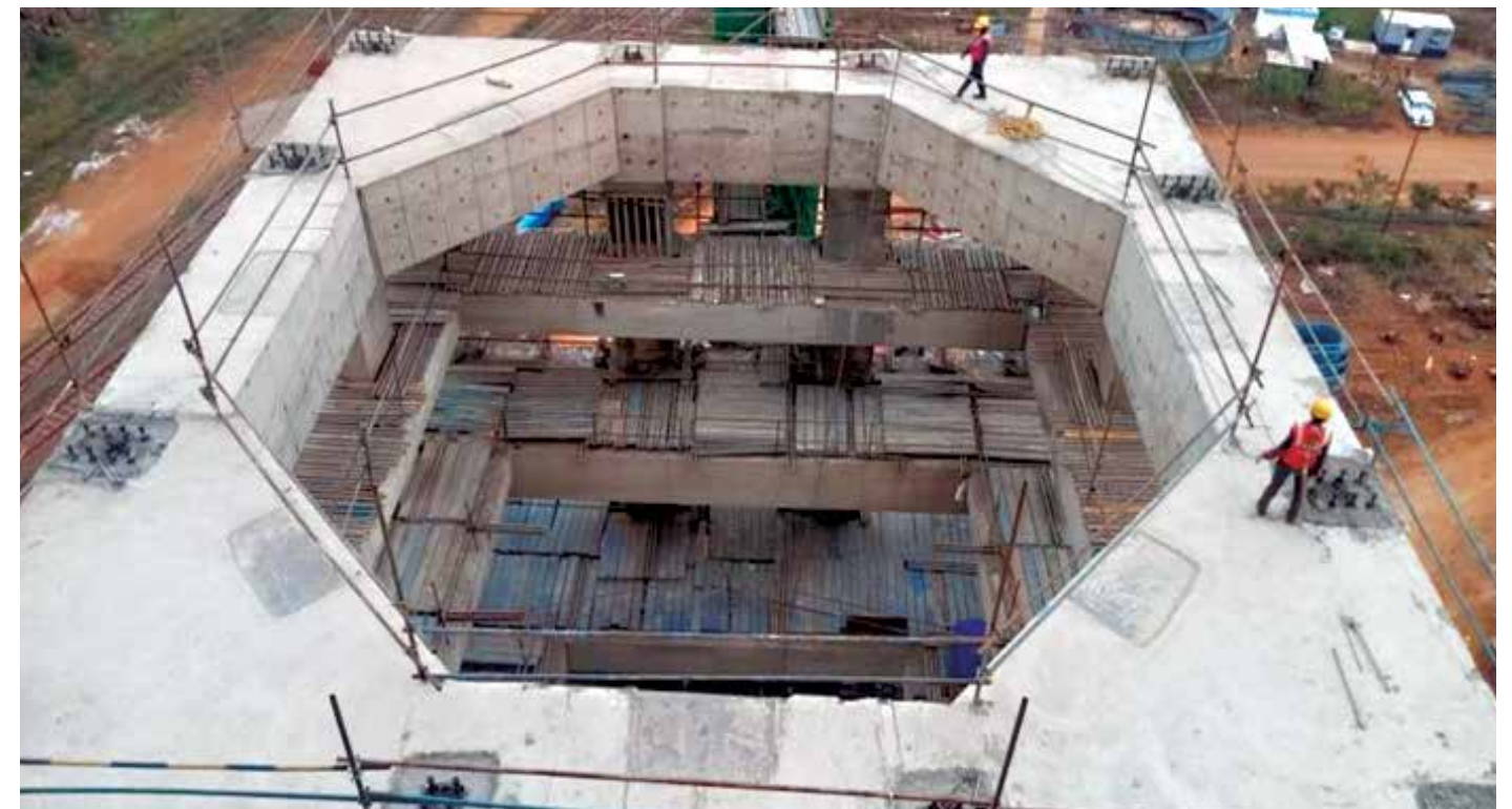
Top view of the Feedbin building at the Utkal Alumina Expansion project
