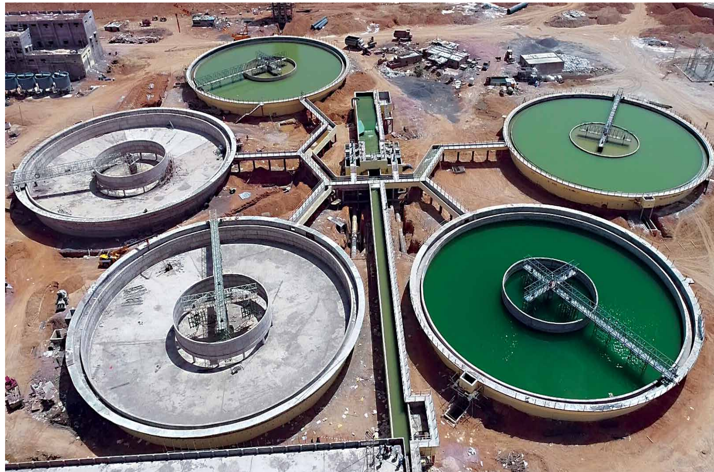
Inlet and Clariflocculator Unit
