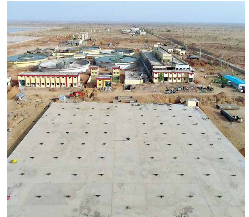
250 MLD Water Treatment Plant at Nokhadiaya
