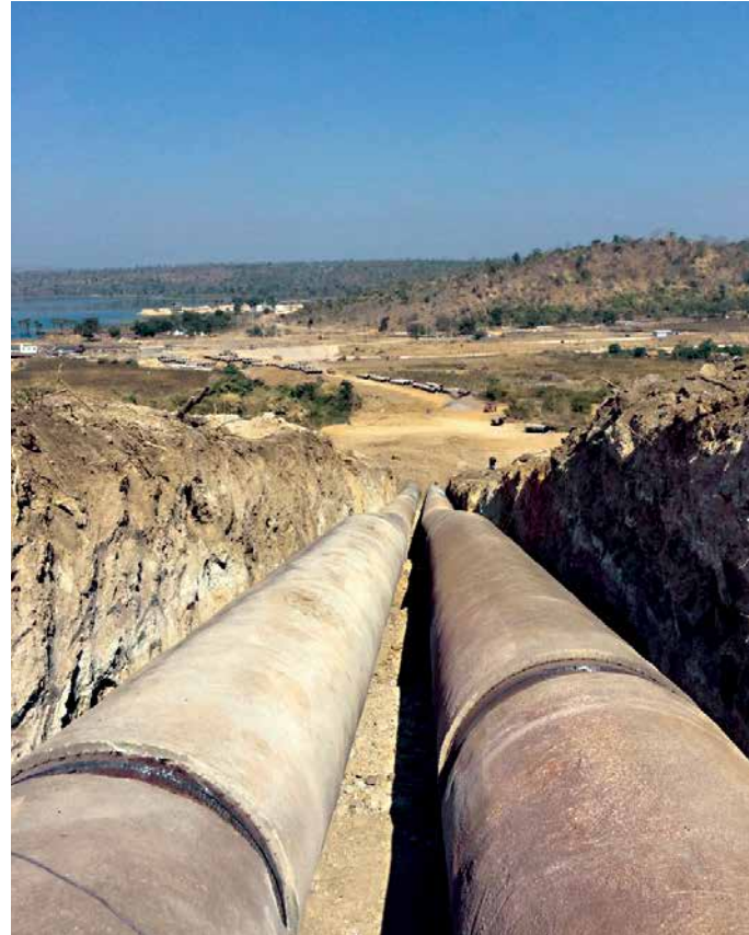
MS Pipeline (Pumping and Gravity Mains)
