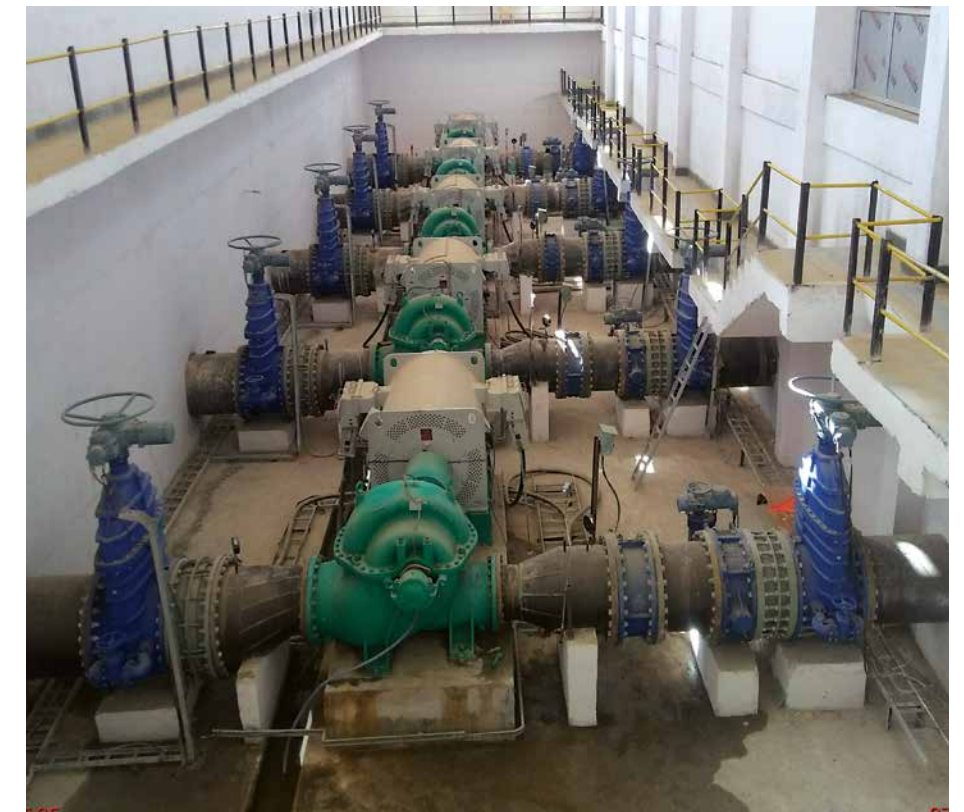
Pumping Station at Deshnok Headwork
