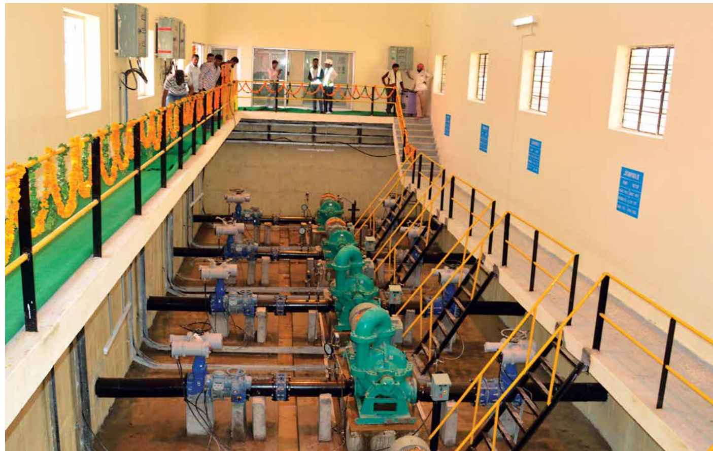
Pumping Station at Jayal Headwork
