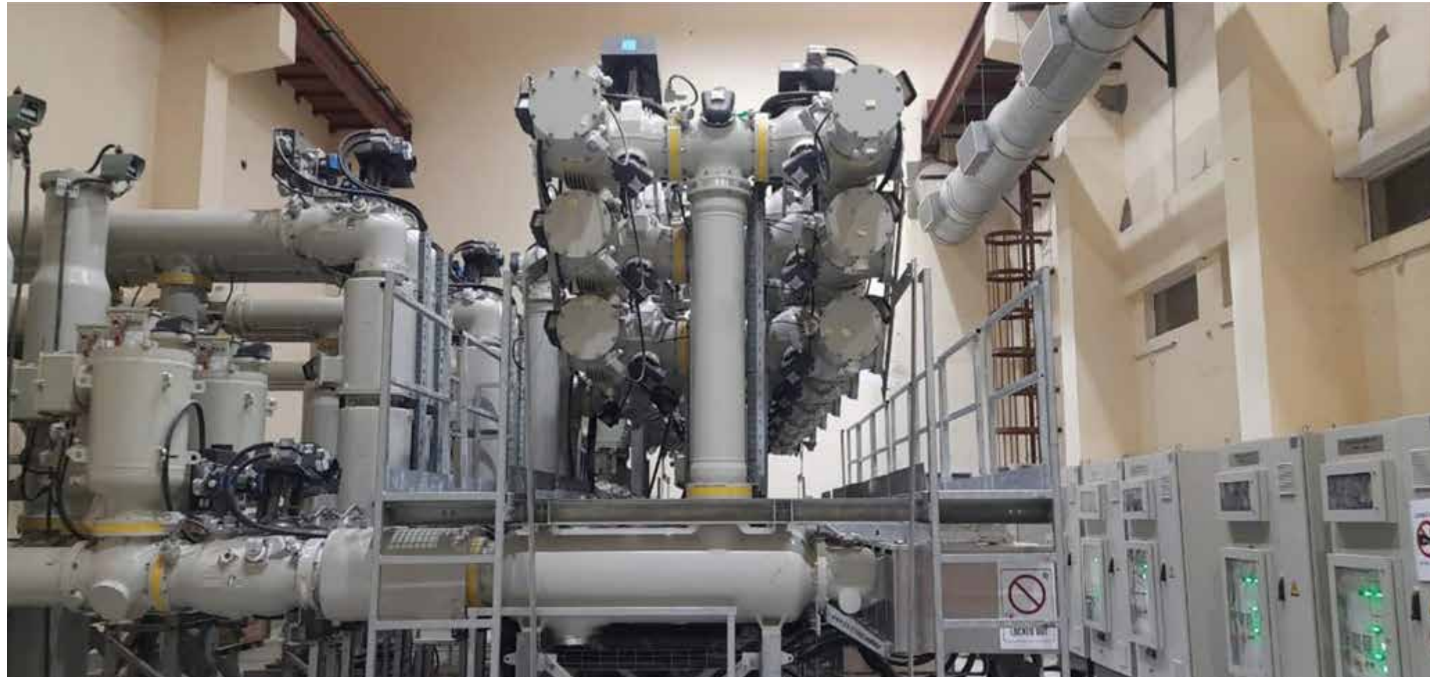
220/33 kV Gas Insulated Substation (GIS), Ranchi
