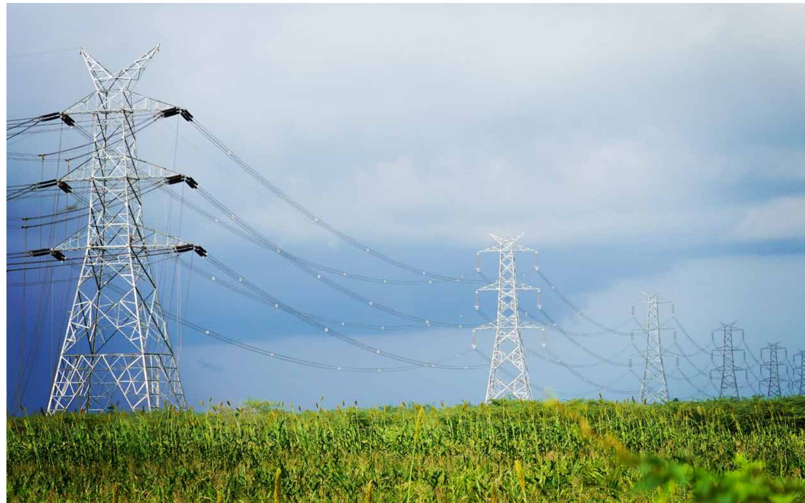
400 kV Kamudhi-Ottapidaram Transmission Line
