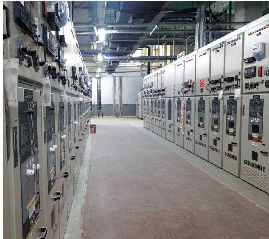
Electrical Room – DIAL T2
