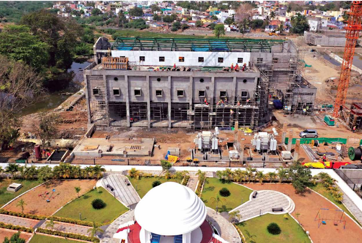
Pump House 1, near Kalingarayan Anaicut, Bhavani
