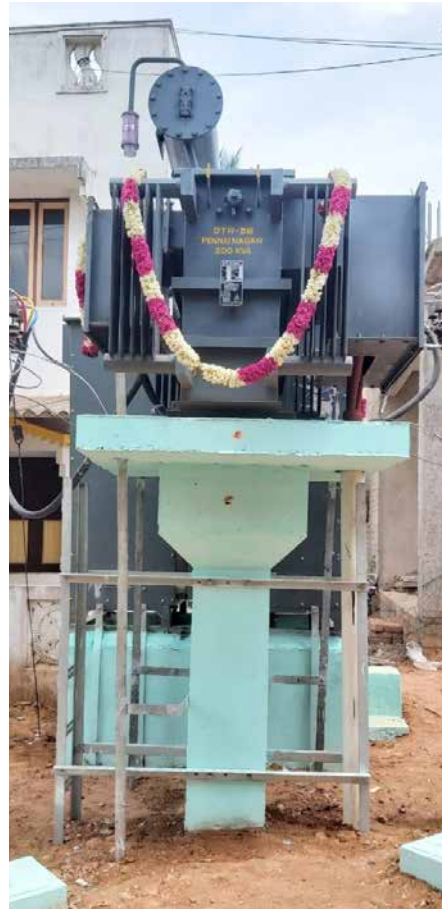
A transformer installed at one of the locations in Cuddalore as a part of the Under Ground Cabling Project
