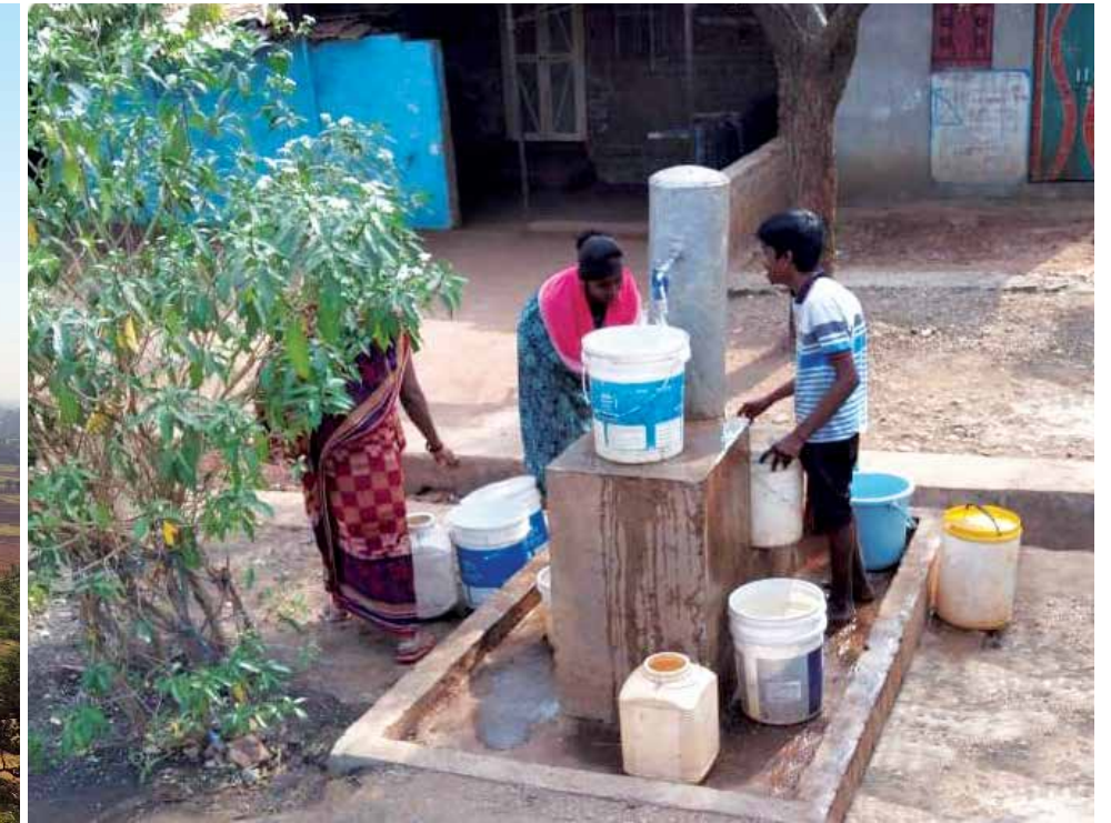
Public stand post for remote location water distribution
