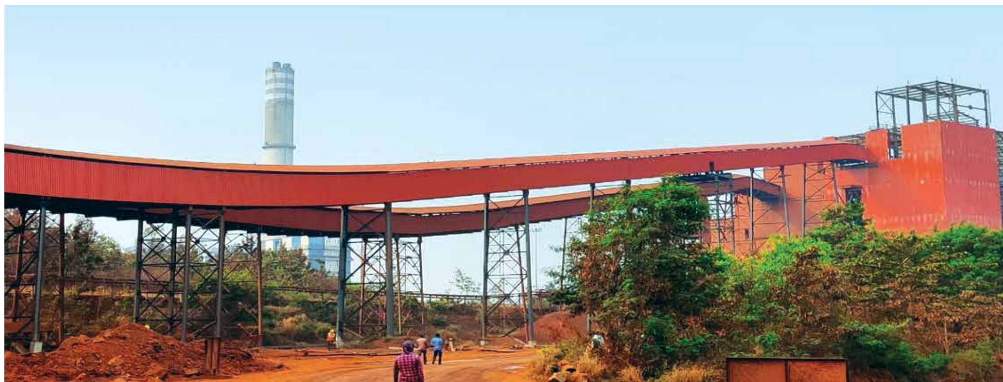
Bauxite Handling Conveyer - UTKAL
