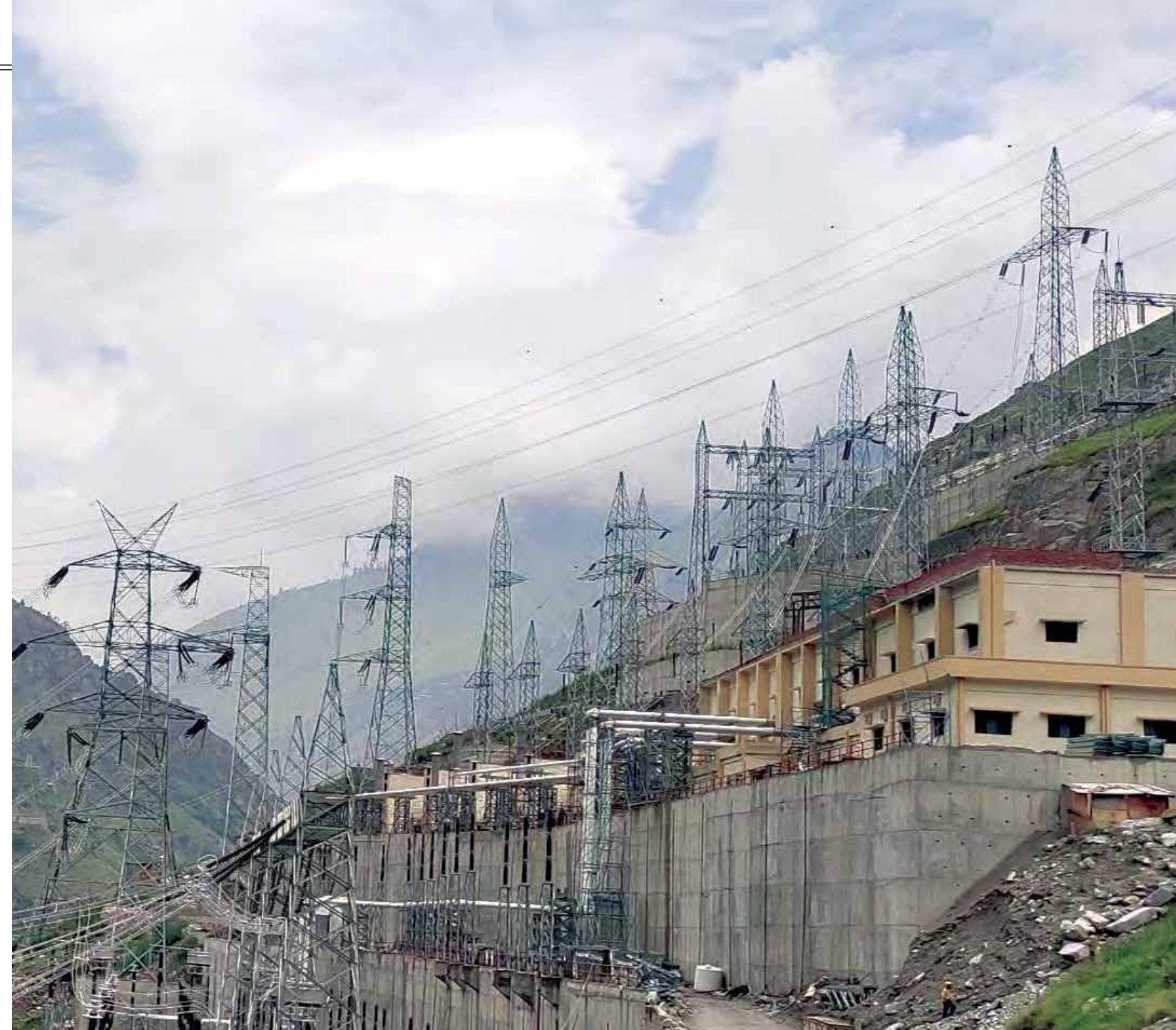
400 kV Wangtu Substation
