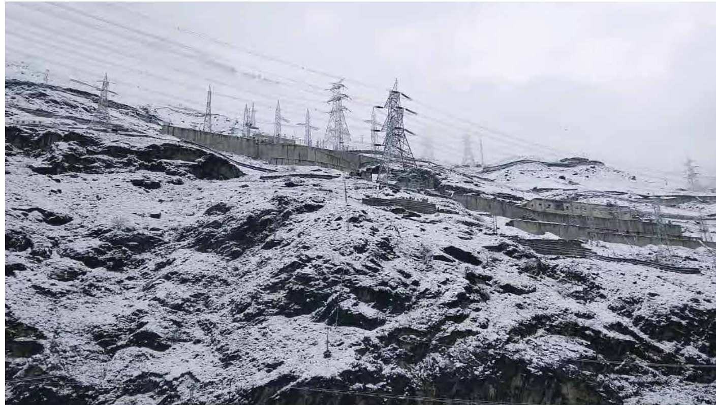
A view of snow clad terrain around the Wangtu Substation
