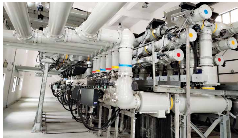
An inside view of the Wangtu GIS
