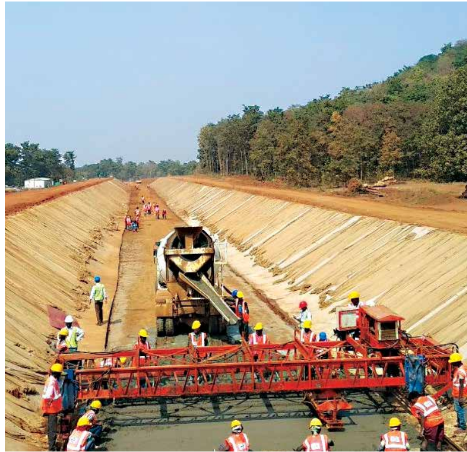
Building a water life line canal with secure sloping and benching methods
