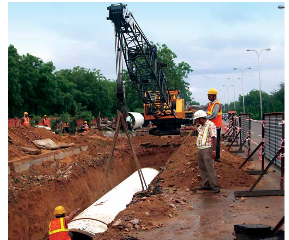
Workmen busy laying pipes under the watchful eyes of supervisors in a well barricaded zone
