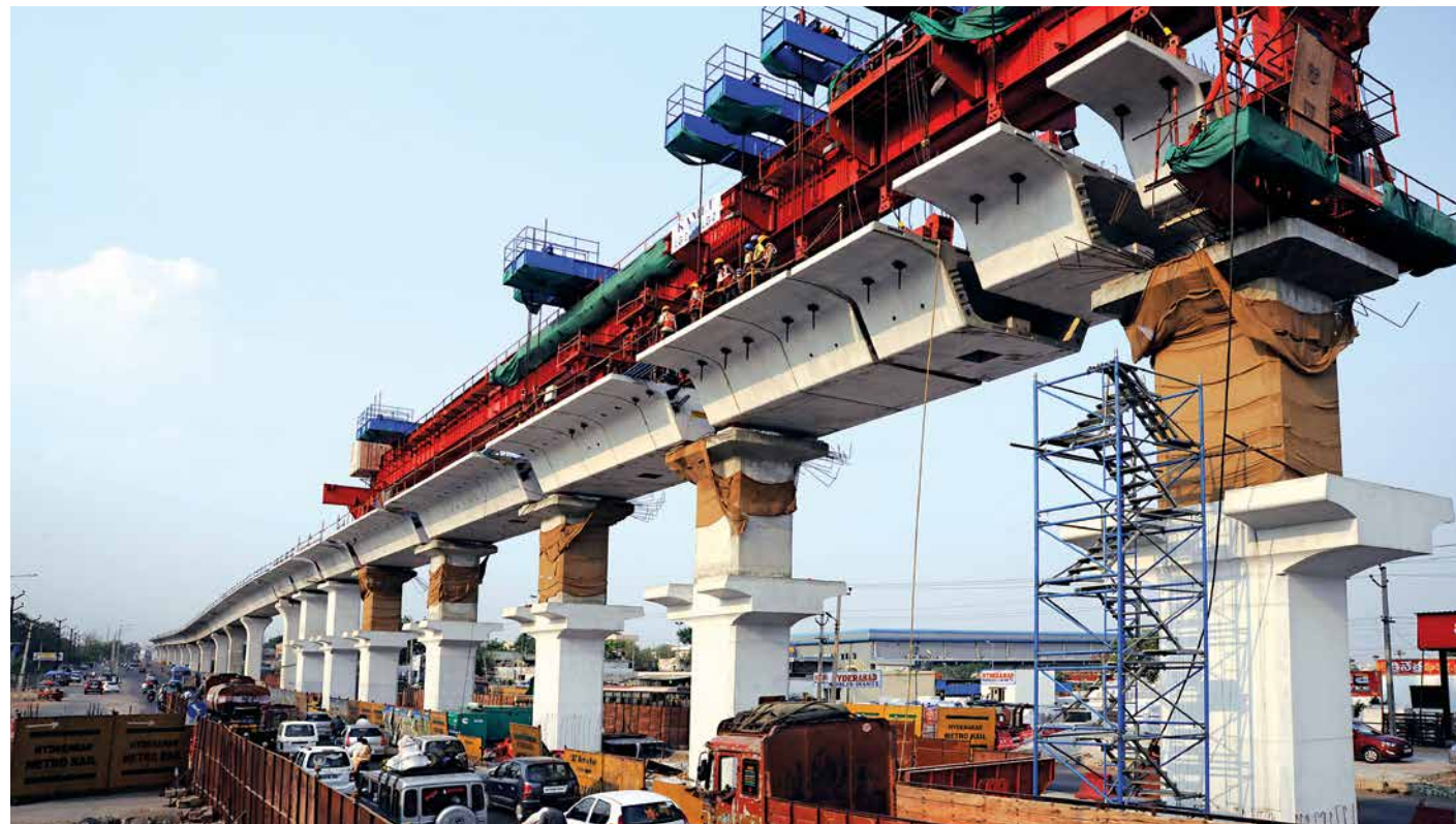
Girder erection using push launch technique with a marked secure zone for vehicle transit
