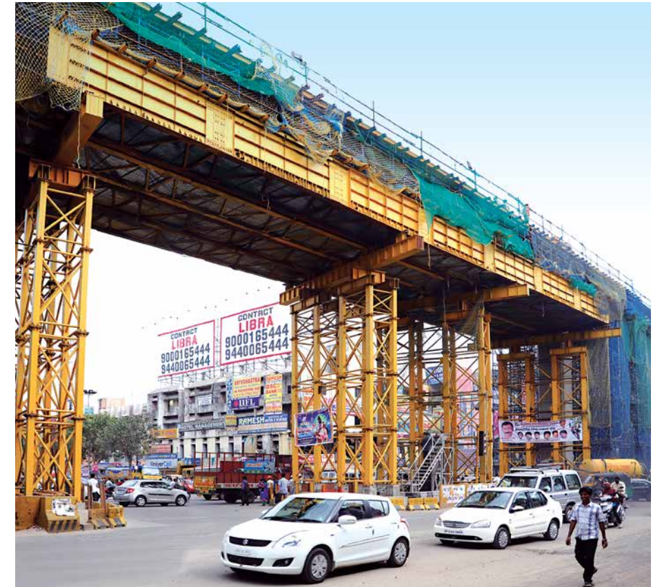
Putting safety first for a steel girder erection across a busy traffic junction
