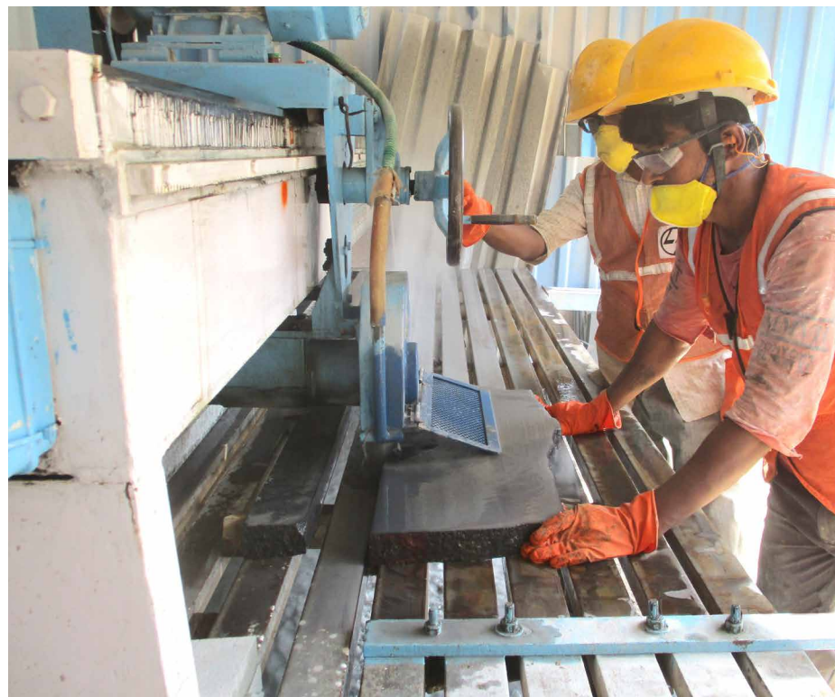
Granite stone cutting machine with customised guards fitted for onsite cutting works
