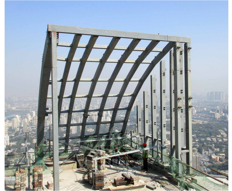
Crown works on the roof of the tower at 225 m above MSL
