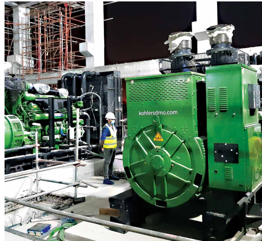
Operations & Maintenance at the Industrial Area Sewage Treatment Plant, Qatar
