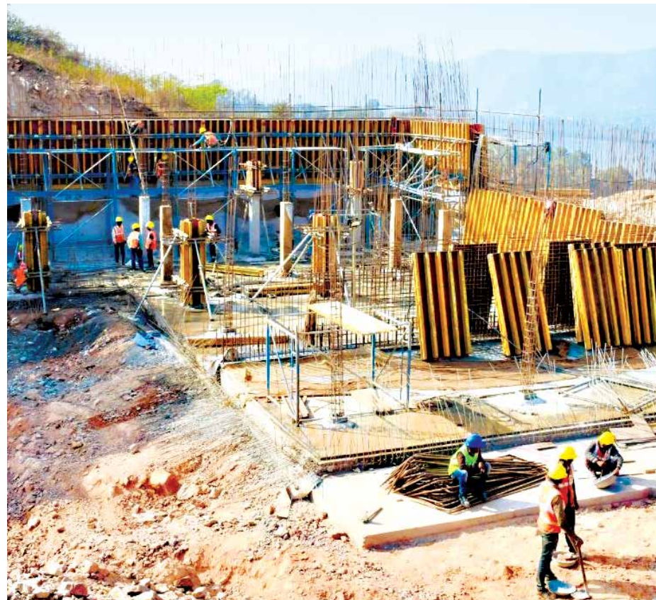
Construction of a WTP over a hill at Udaipur Integrated Infrastructure Project
