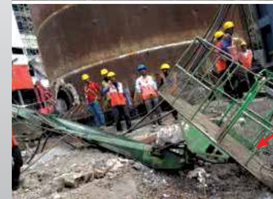
Position of the boom and platform after the fall
