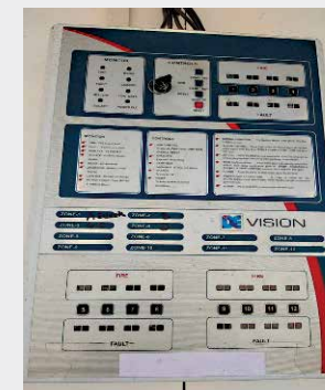
Fire alarm control panel
