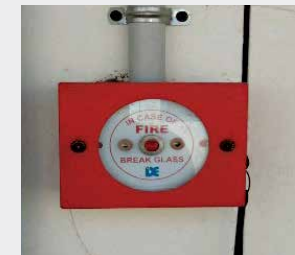
Emergency break glass
