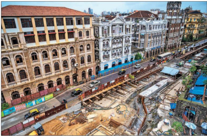
Work in progress on Metro Line 3 and Hutatma Chowk station near Flora Fountain.
