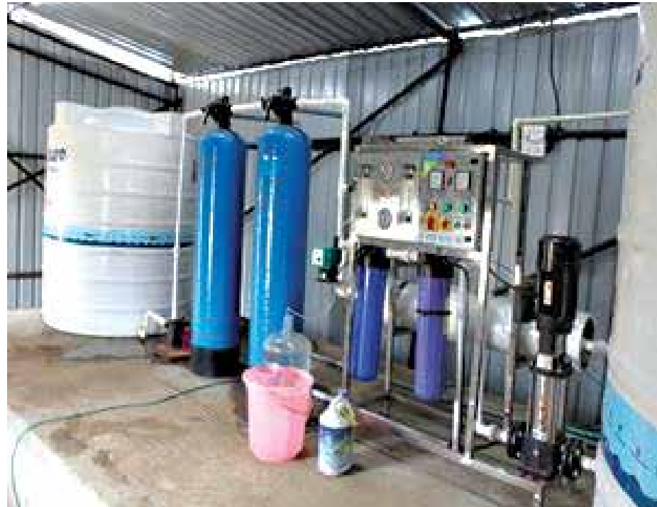
RO Plant installed at site
