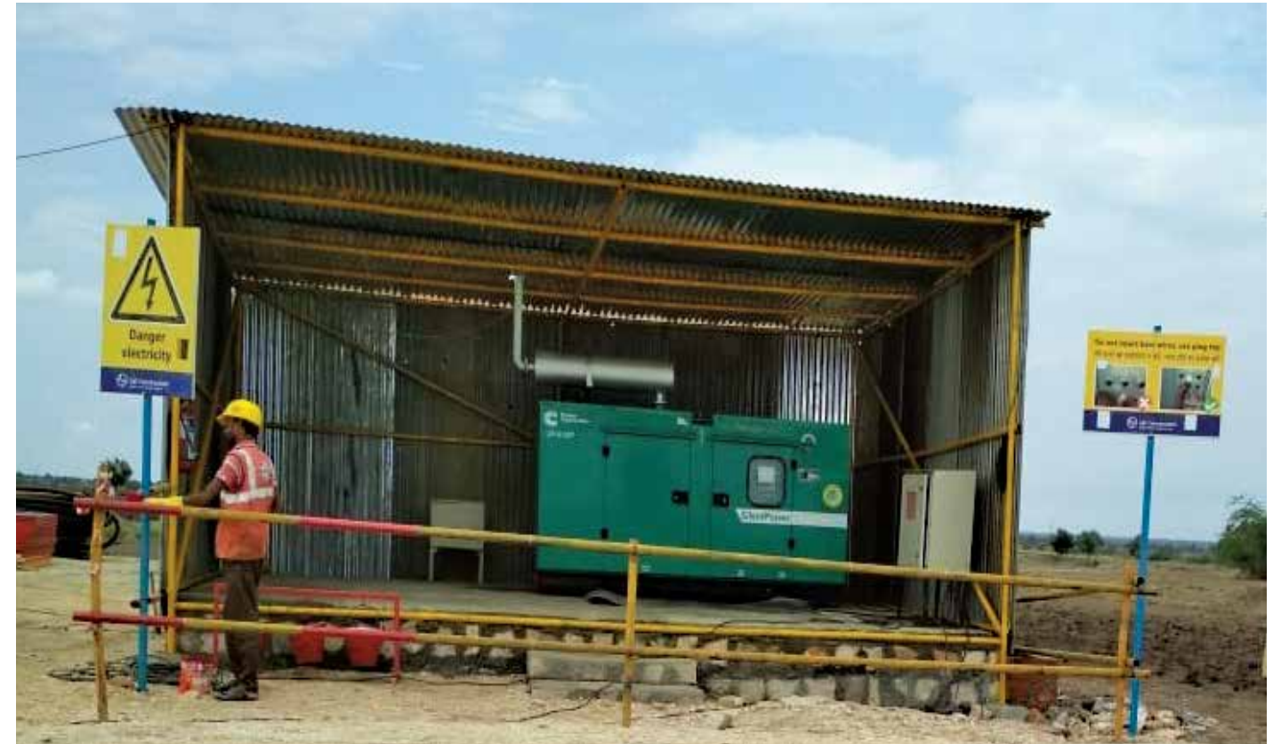
Power generator installed on fabricated stack to ensure soil protection
