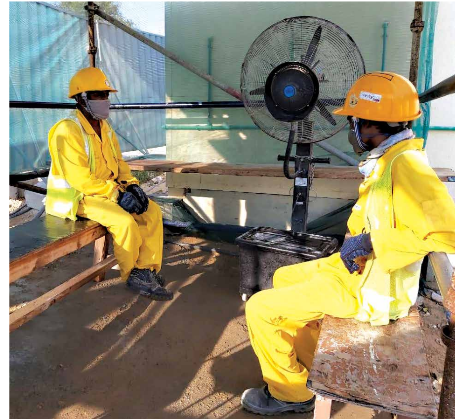
Misting fan installed at shading sheds
