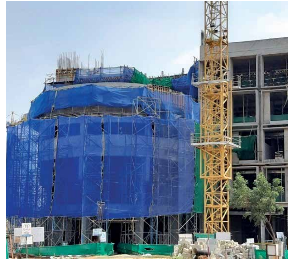
A vertical safety net around a circular building
