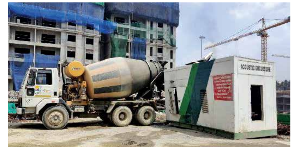
An acoustic enclosure around a concrete pump to arrest noise
